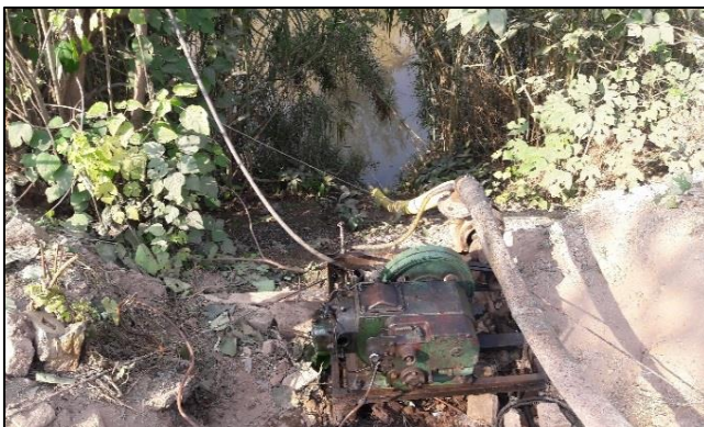
Fig. 2: Pumping of sewage water used for irrigation at Tarlai farms.
