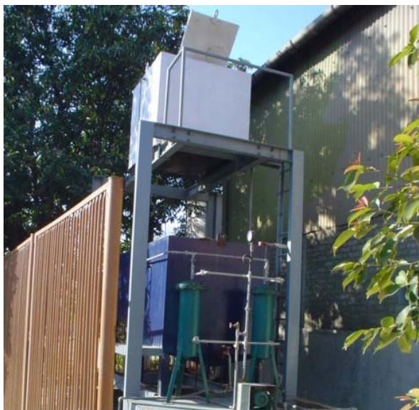
Car wash waste water recycling.
