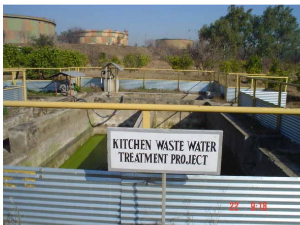
Kitchen waste water treatment project at ARL
